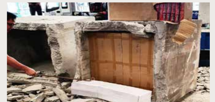
A mini excavator was used to hack the concrete blocks to retrieve the duty-unpaid cigarettes concealed within it.
